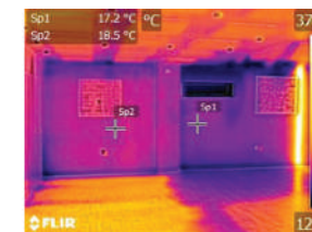
[Before] - Showing western extent of 'eco' wall at wall pier in centre of image. Note that the 'eco' wall (Sp2) is 3.3°C colder than the extension to the left of the pier (Sp1). Both images show considerable heat loss (thermal or cold bridges) at the wall ceiling interface.
