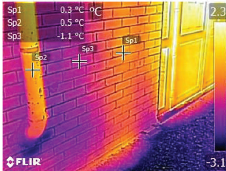
[Before] – Former soil vent pipe (SVP) much warmer than external face of wall – losing heat to outside. Appear to have been blanked off with plasterboard but not thermally insulated. Location of UFH pipes clearly visible|
