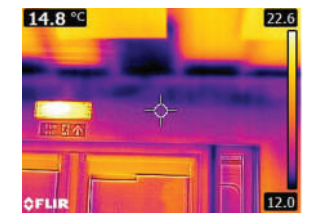
[Before] - Wall open temp is 14.8°C i.e. 4°C colder than ambient temp. Note cold bridging at wall ceiling interface.
